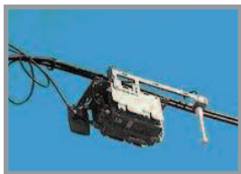
FIGURE 2: Wi-Fi access point suspended on an aerial cable TV line
