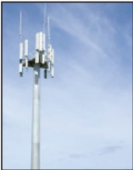
FIGURE 1: Macrocell site tower and base station
