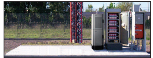
New Network Vision Multi-mode Base Station
