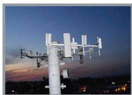
Verizon antenna for 700 Mhz/LTE site
